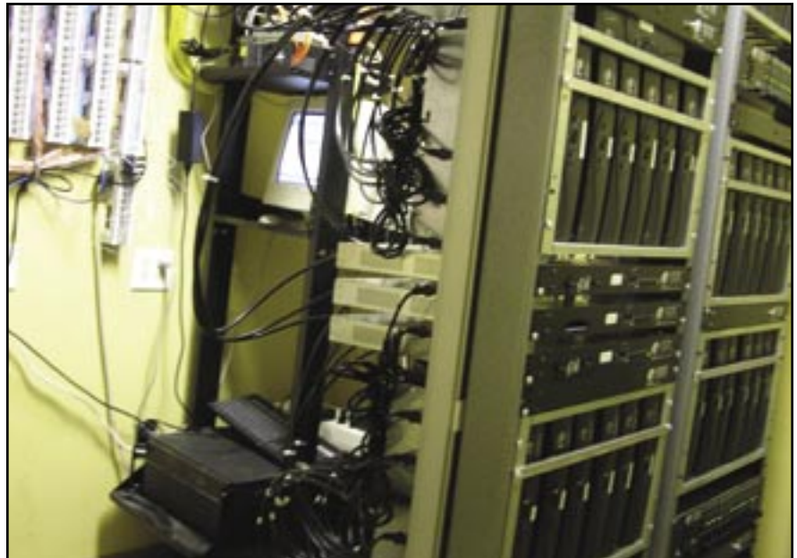
Proper planning and design at the headend can save both time and money.
