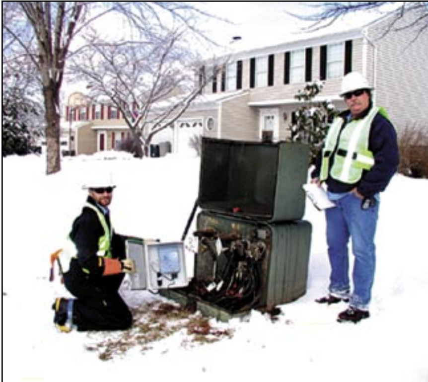
Two City of Manassas employees at an HFBPL node, a transformer where the fiber and BPL networks meet. Each node location services anywhere from 10 to 40 customers with BPL.
