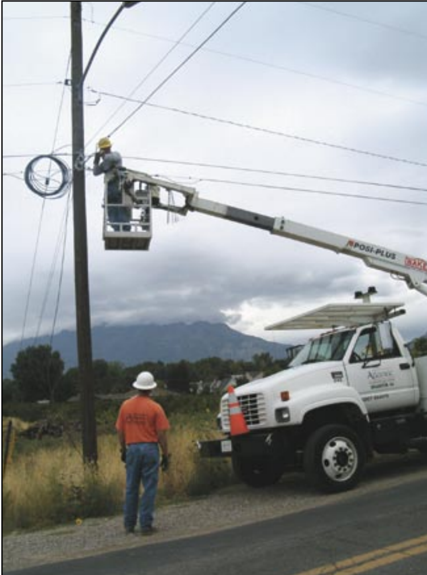
Provo uses a combination of underground and aerial wiring. The customer premises equipment, concentrators, and access distributors are from World Wide Packets. Atlantic Engineering is the contractor.
