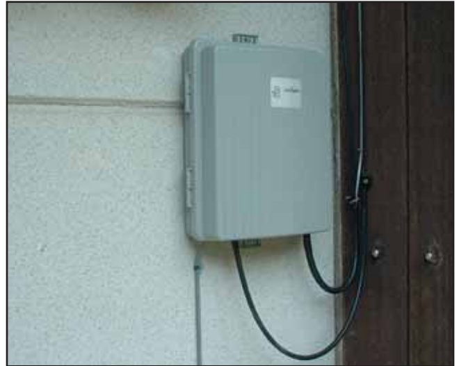
Customer-home installation in Japan, using Wave7-Hitachi AMN1200 equipment for triple-play; note multiple connections.
