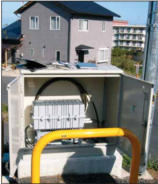
Wave7 Optics Last Mile Core OLT installed at roadside (hence the protective bars) in the Taki-Cho project in Japan.
