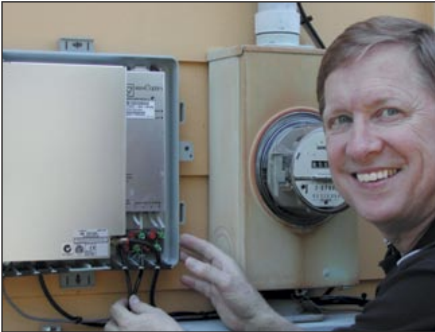
Broadband connection at side of home; inside, residents see an Ethernet jack.
