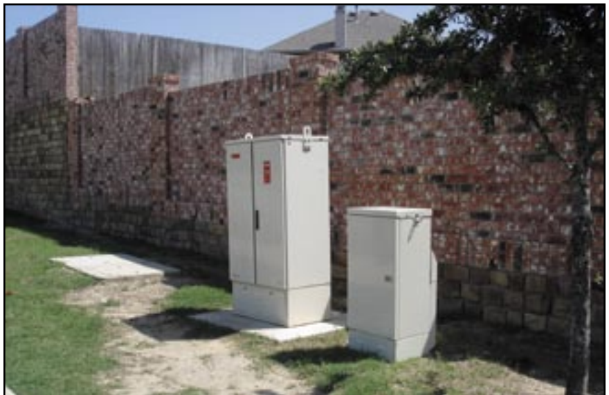
Figure 1 - Reduced-size local convergence point cabinet (right), full-size LCP (left).
