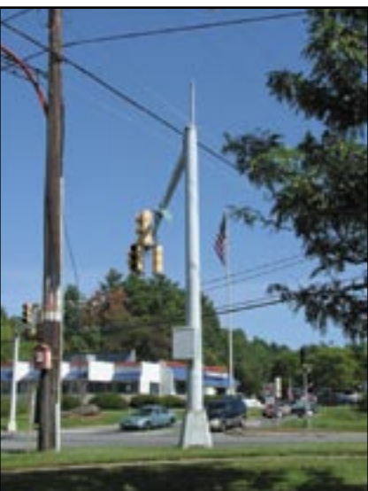
Figure 2: The new look of cell sites – telephone and utility poles.
