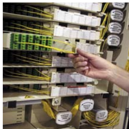
Note the modular drawers in Tyco’s design, and the fiber “parking areas” to the left.
