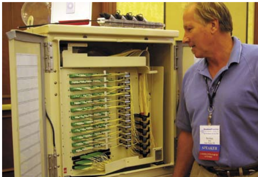
Fiber pioneer Pat Sims shows off ADC FDH with angled splitter trays and error-resistant spools.
