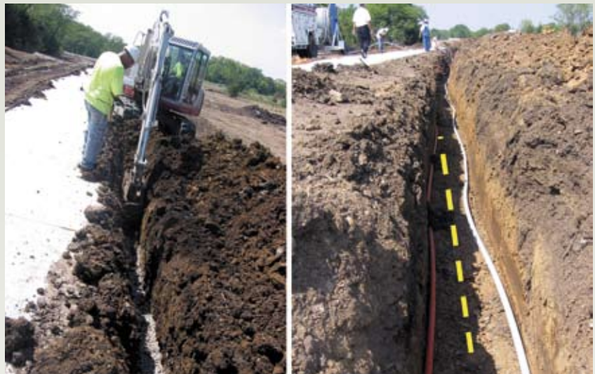
Trenching for fiber conduit installation. Example of co-location of power and FTTH in a private easement adjacent to a public easement at Rockfire at the Lake.
