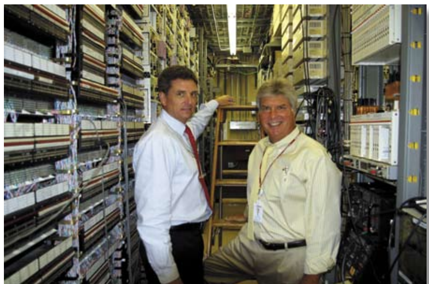
Willy Pirtle, VP sales (left) and Rich Church, business development manager, at Shentel's switch room.
