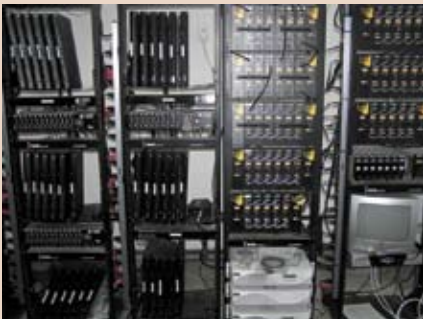
Video headend racks in on-site central office.
