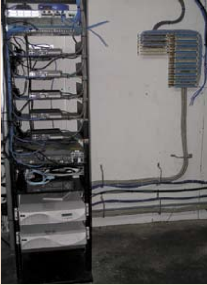
The VoIP rack in on-site central office.
