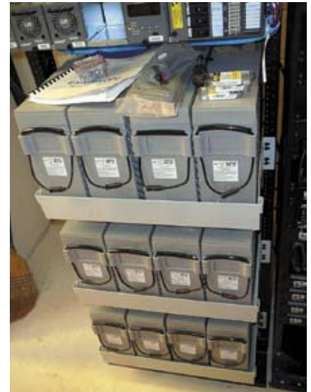
UPS batteries for emergency power supply within the on-site central office.
