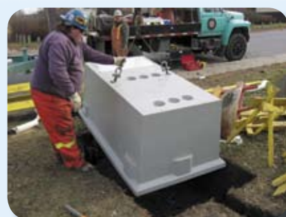
A polymer concrete cable vault.
