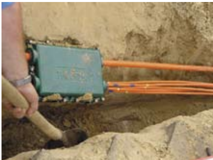
Figure 5. Buried microduct in Nuenen, in the Netherlands. Microduct containing the main fiber is at top; smaller cables for homes fan out from junction box below.
