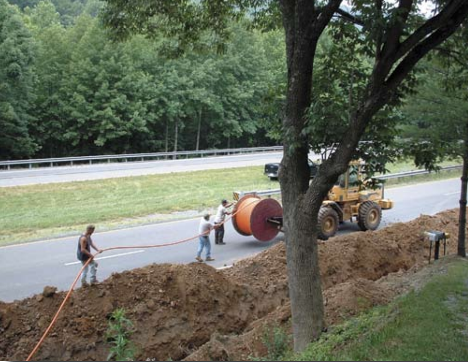
Figure 3. Unspooling microduct for a roadside installation. Here, underground ducts were necessary because there was no existing aerial telephone or power line over which to string fiber. The fiber cable itself is considerably less bulky.
