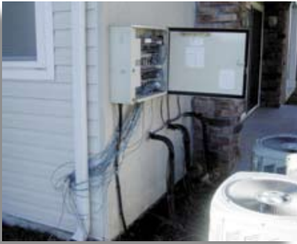
Problematic cable management and organization at demarcation point.
