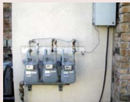
Precarious grounding and lightning protection daisy-chained to incoming natural gas meters by MSO's installer.
