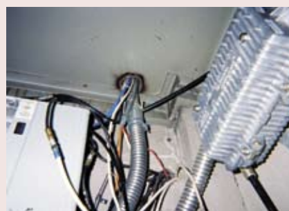
Ill-fated penetration of 4-hour-rated stairwell ceiling and walls without assembly or fire-resistant seal.
