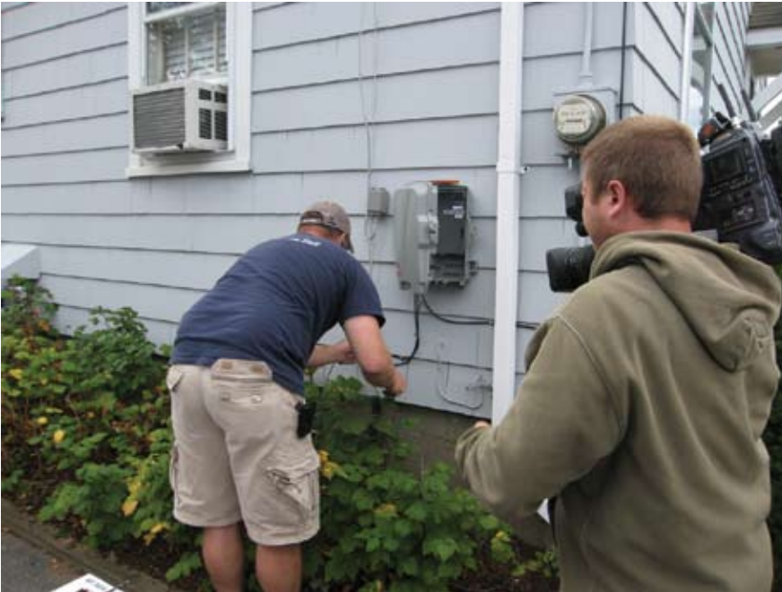
BT workers install an optical network terminal at the home of the 2000th subscriber.
