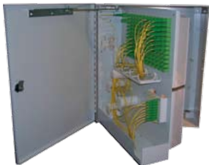
Figure 3. EZ-Plug fiber distribution hub.
