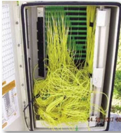
Fig. 3. Disorganized fiber splitter cabinet.
