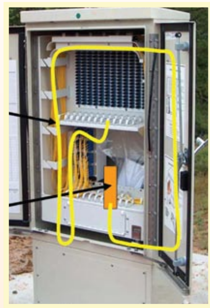
Figure 4. Fiber distribution hub with traditional rectangular fiber management.
