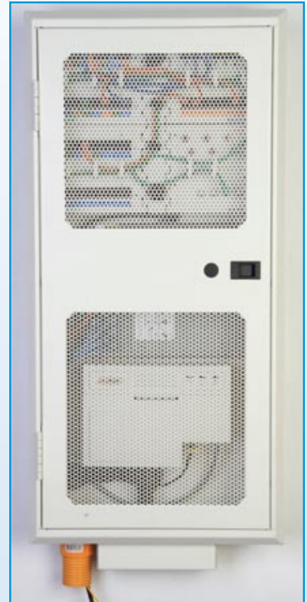
A perforated door protects components in the structured cabling panel while also enabling passive cooling.
