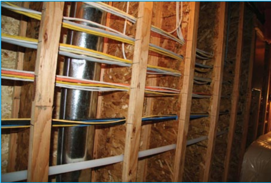
Example of “home run” wiring in the studs of a wall. This approach helps to ensure maximum bandwidth and ongoing reliability.
