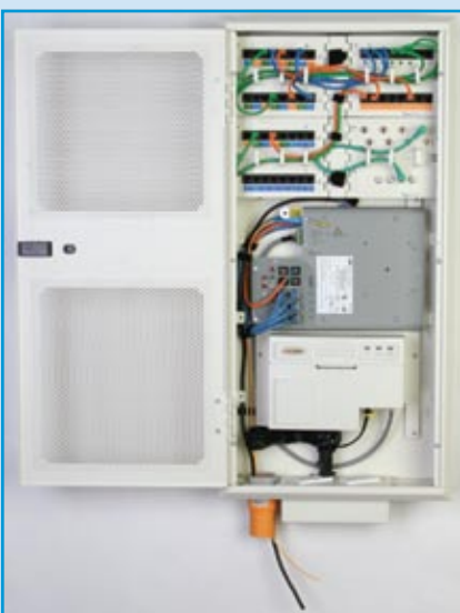
A fully installed home structured cabling panel. Note the space in the lower half of the panel for routers and other active equipment.
